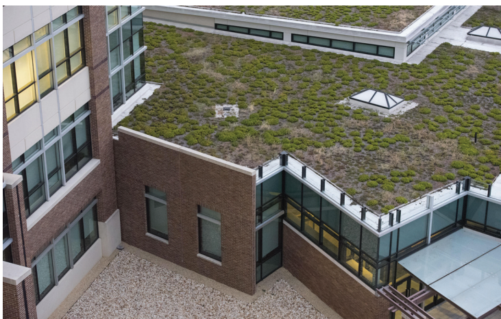
Figure 9.4: Living roof on a building at the US Air Force Joint Base Andrews, MD.
